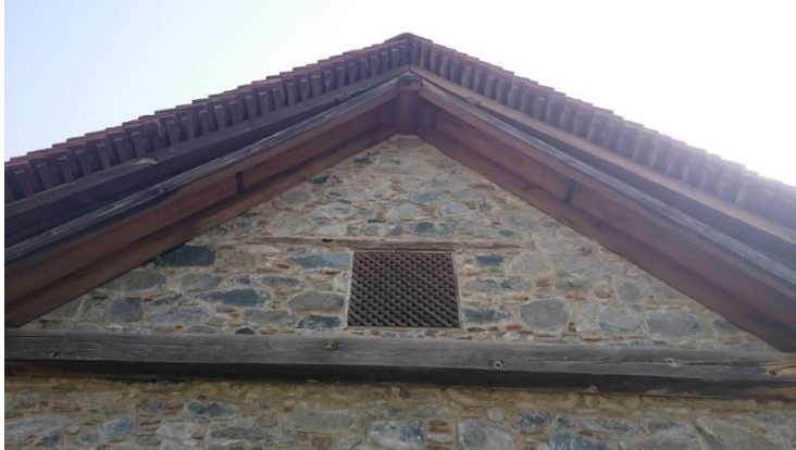
fig. 5.7 One of the two pediments of the church at Moutoullas with the wall plates and the masonry being constructed until the top following the steep angle of the roof
