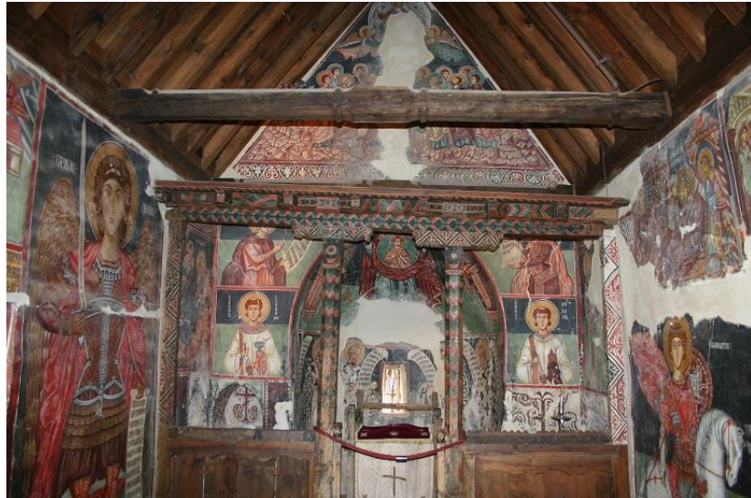
fig. 3.5 View from the inside showing the tie-beams that connect horizontally the wall plates together
