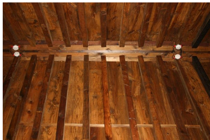
fig. 3.8 The rafters holding the planks and the ridge-purlin on the highest part of the internal roof
